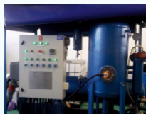
Oil reconditioning machine
